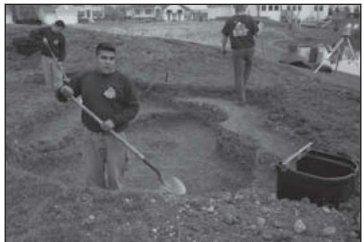
Fig. 7 Dig the pond to its max depth and finish excavation of the skimmer hole.
