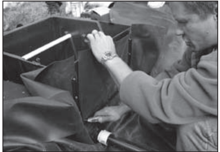
Fig. 16 With all of the screws started, cut the liner using the inside of the "U" frame as a guide.
