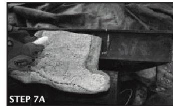
STEP 7A Fig. 12 Decide where and how wide the waterfall stone will be and cut the vault to match.
