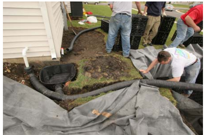
Downspout Filter located under roof's gutter system for collection of rainwater run-off. Piping connected from Filter to storage basin.
