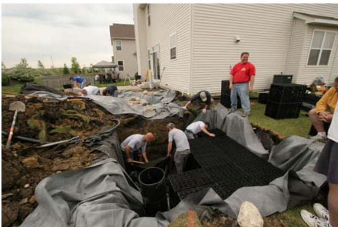
Forty modular AquaBlox® set into excavated storage basin after liner is laid into place. Up to 1300 gallons can be stored underground.
