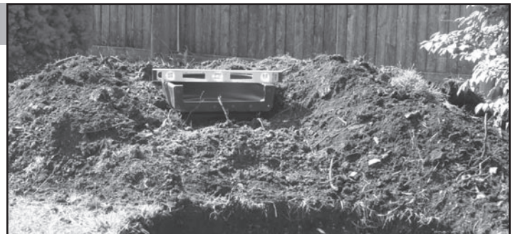
Fig. 5 Soil backfilled around the BIOFALLS® filter helps hide the filter and creates a planting berm.
